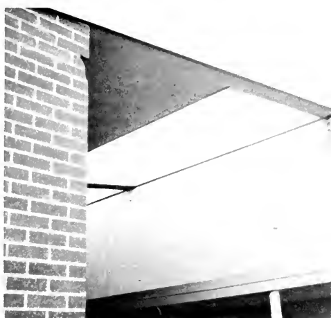
Photo 20. Soledad Canyon Elementary School. Damage in reinforced grouted brick masonry wall below roof beam at left.
